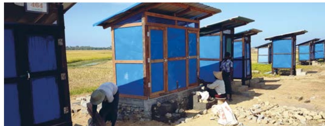
Image description: People constructing a row of toilet units. Credit: Bagus Setyawan/Oxfam.
