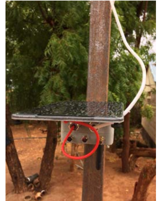
Image description: A small box with wires coming out of it and a solar panel above it sits attached to a metal stake. Credit: BRCK.
